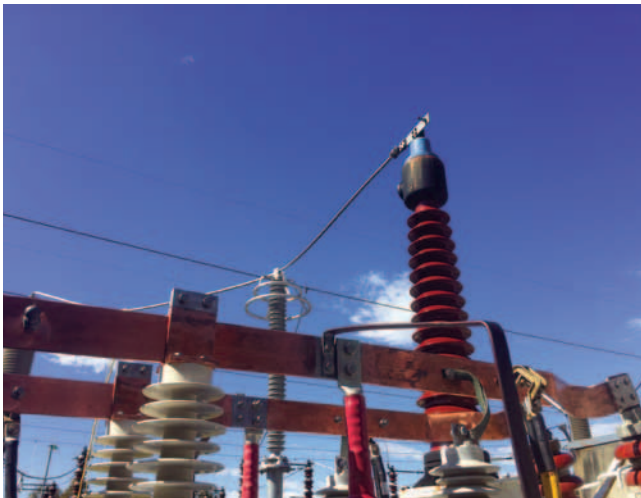
Transformer cable connections.
