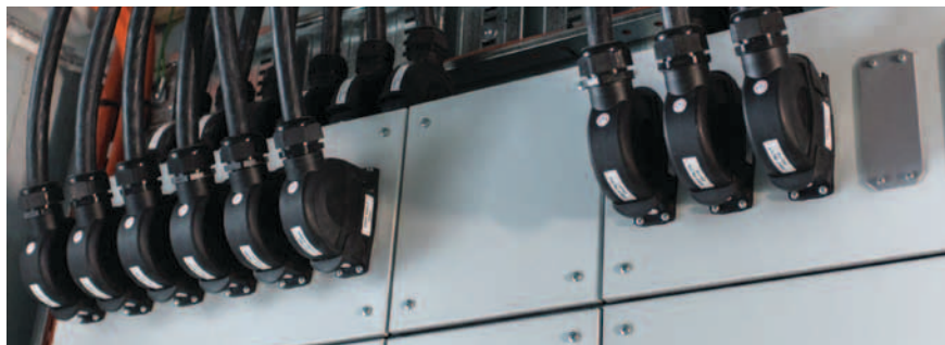
Modular wiring uses the same principles as the automotive wiring harness.
