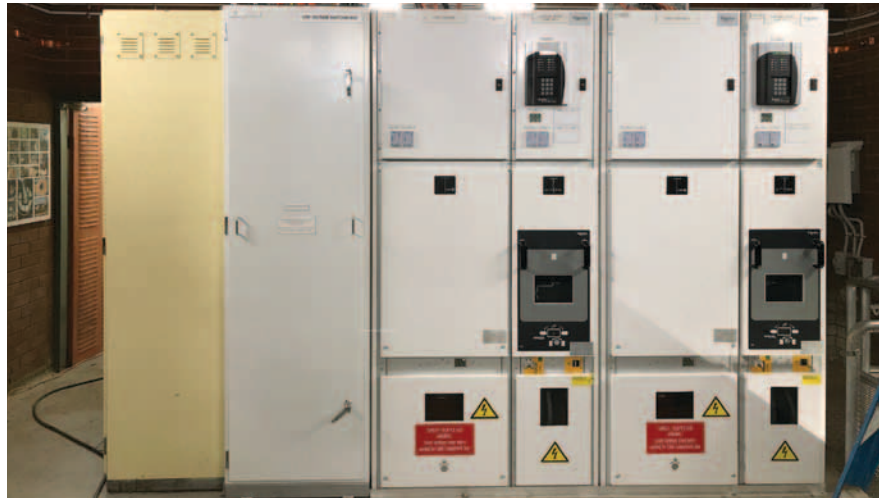
New HV SWB and SCADA panels were installed for the Capation Cook Memorial Jet.
