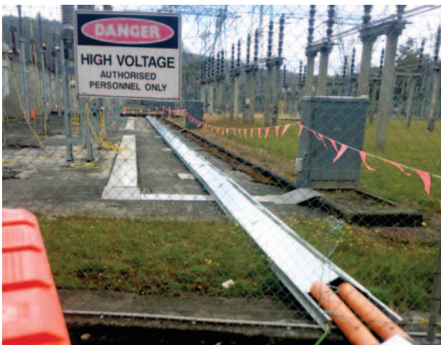
RBD replaced the three hydro 31MVA generator set 11kV power cables from each generator termination to each switchyard power transformer termination.
