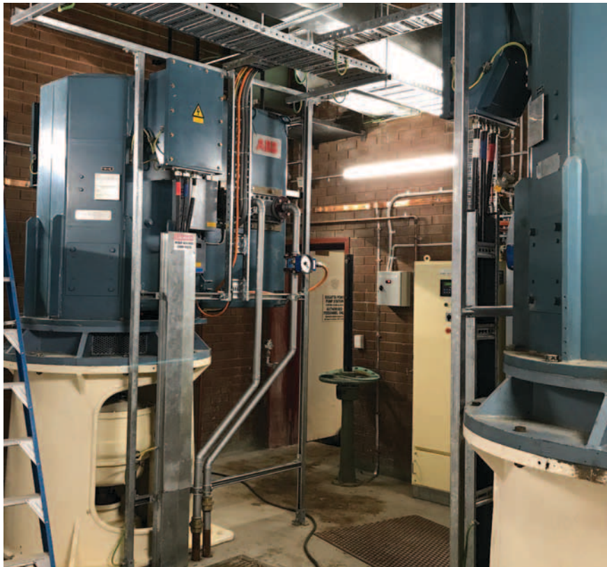
Shepherd Electrical installed new cable tray as well as new high voltage cabling.
