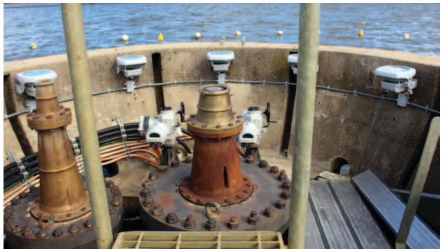
The Captain Cook Memorial Jet saw a number of new lights installed.
