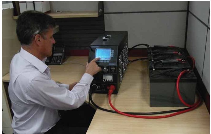
Figure 1: The state of charge of VRLA batteries being checked on an IDCE840 battery tester. Image courtesy of Power Parameters.
