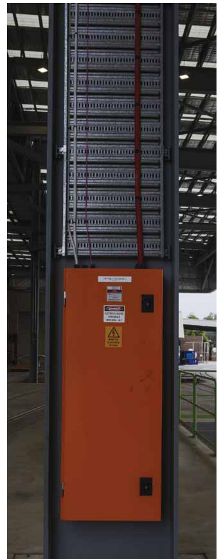
Kerfoot had to install a new power supply connection for Plasser Australia.
