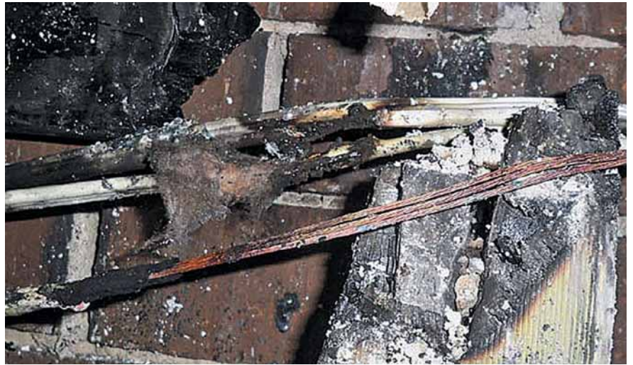
Fire damage near a particular wall stud.
