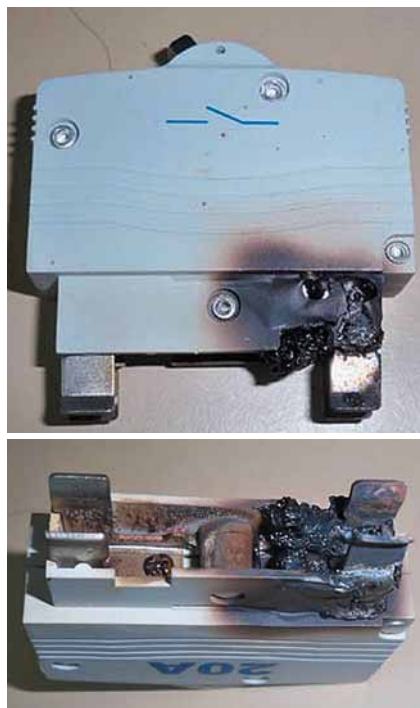
A plug-in circuit breaker that has caught fire due to a high-resistance joint.
